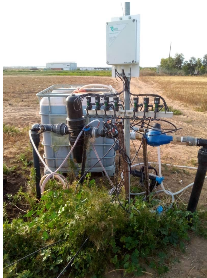
An irrigation network control center
